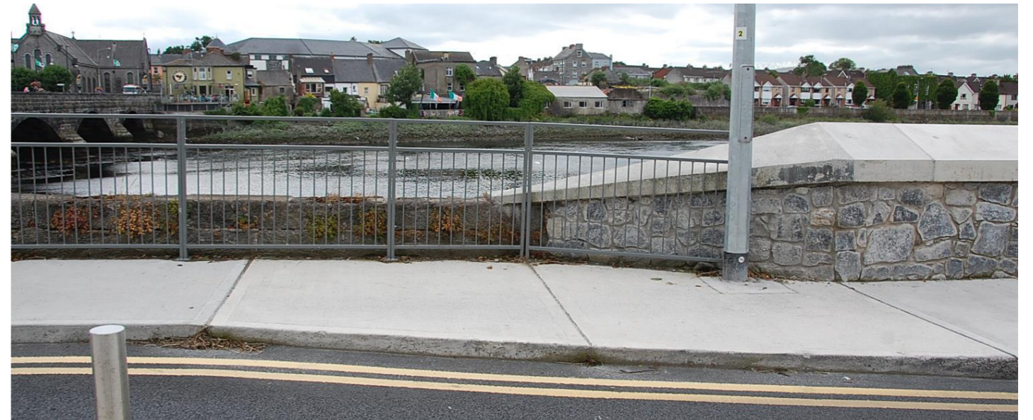
Existing view of the dry-side of the upgraded wall and the existing low wall with safety railing to front.
