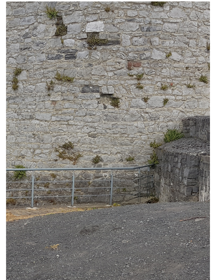
The proposed glass panels will tie into the wall just south of the Castle and the existing railing tie in.
